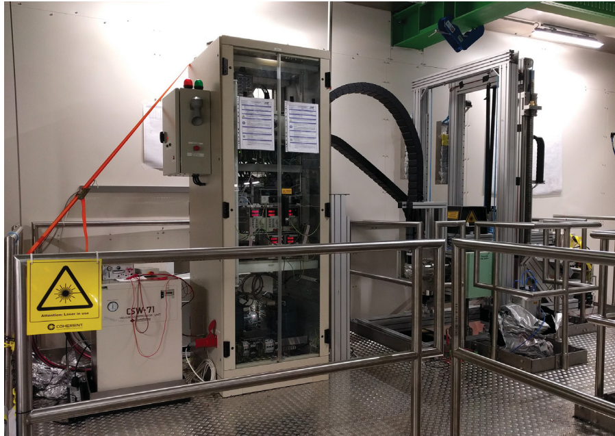
Figure 5.9: CKrS set-up integrated in KATRIN beamline. The complete CKrS is situated on a platform, on top of the CPS. The left-hand side shows the high voltage cabinet, which houses the read-out electronics for ellipsometry, temperature monitoring and control of the gas system. On the right side, the upper CKrS scaffold is shown with the lowered carriages.
