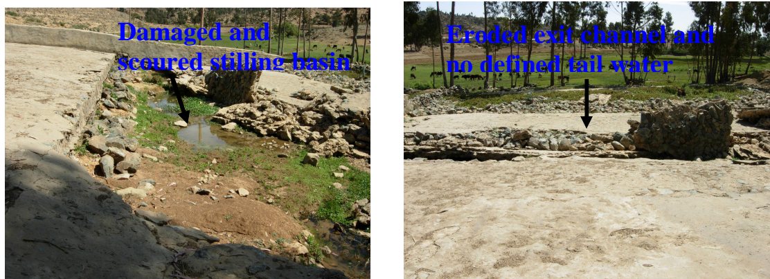
Figure 2-6: Terminal structure failures in Rubafeleg dam
