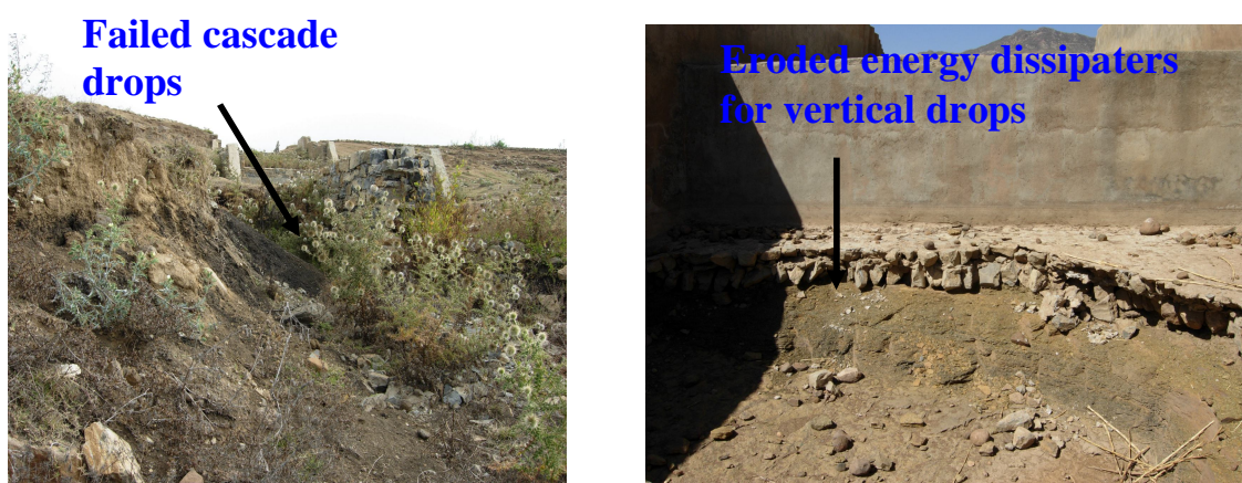
Figure 2-7: Vertical drop spillway failures
